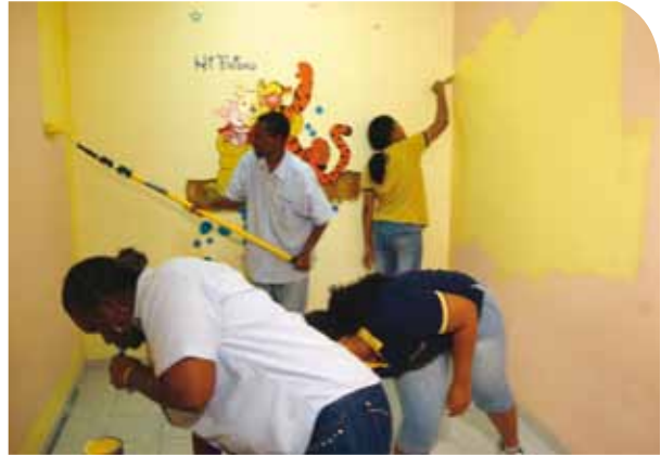
Belize City teams decided to combine their efforts for Adopt-a-Cause. It was agreed to renovate the right wing of the paediatric ward of the Karl Heusner Memorial Hospital (KMH).
